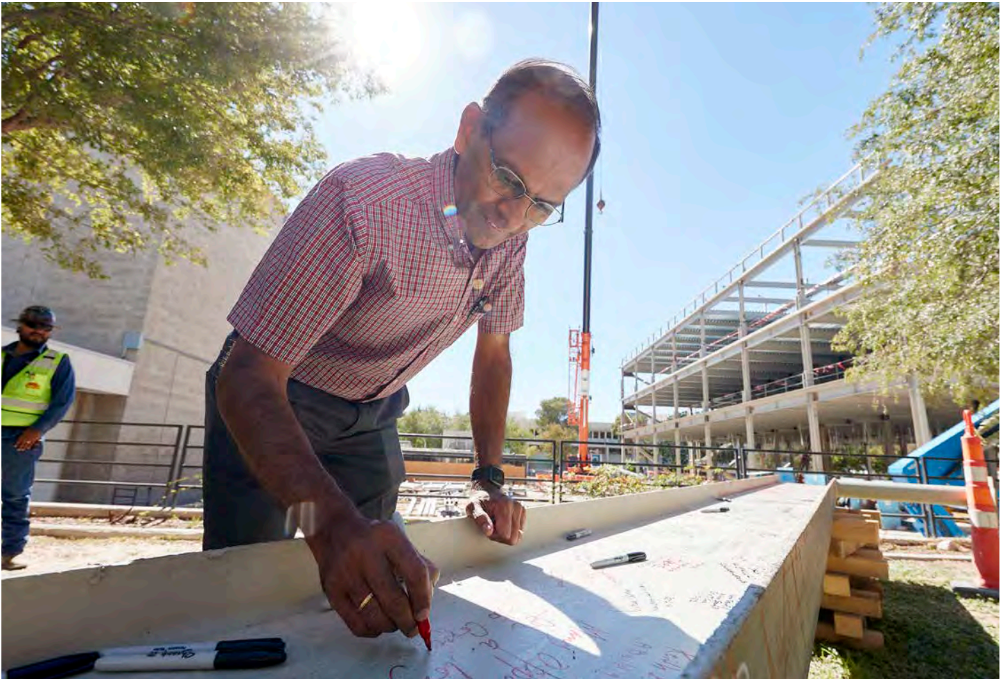
Rama Venkat, dean of the Howard R. Hughes College of Engineering, adds his name to a steel beam before it is hoisted into place at the Advanced Engineering Building, now under construction. Donors, faculty, and staff were all invited to sign the ceremonial beam that became part of the structural support of the new building and the College of Engineering's future.
